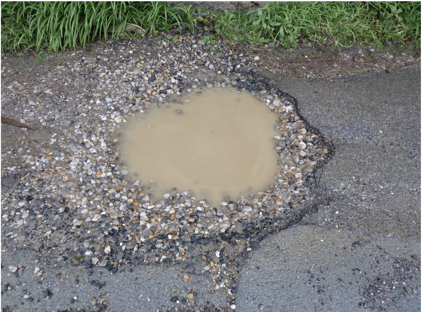
Potholes - damaging to your car and your wallet! Photograph © Kim Henson.
